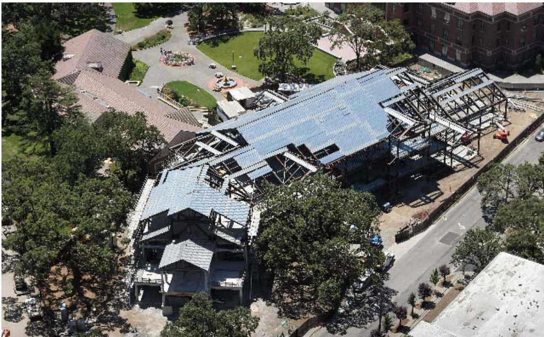
Aerial view of the Bertolini Student Center after structural steel is completed
